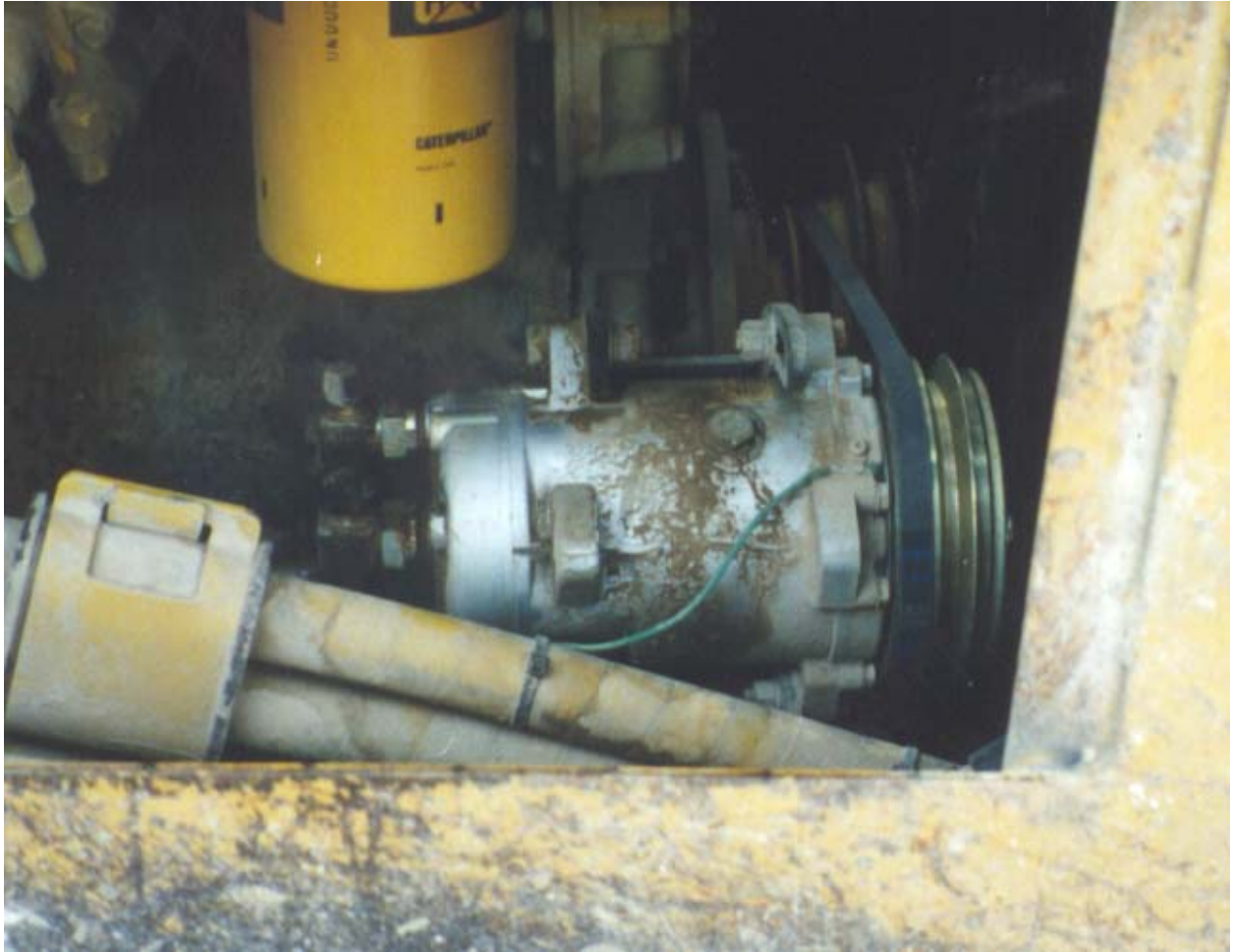
Compressor mounted in place - new style compressor.
