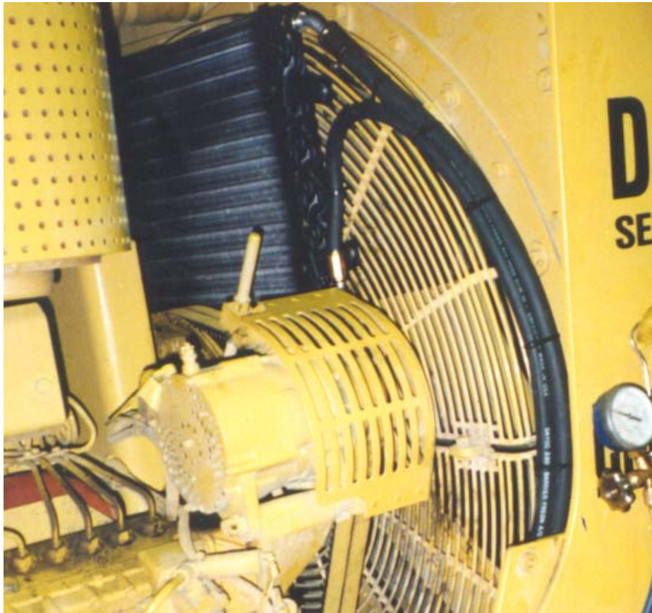
Condenser hose routing down fan screen.
